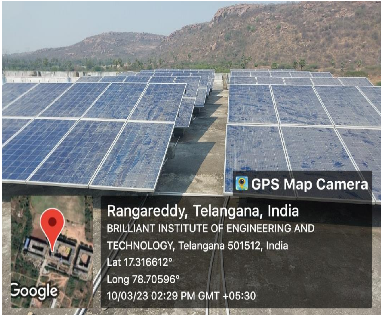
View of Solar Power plant 75 KWp.
